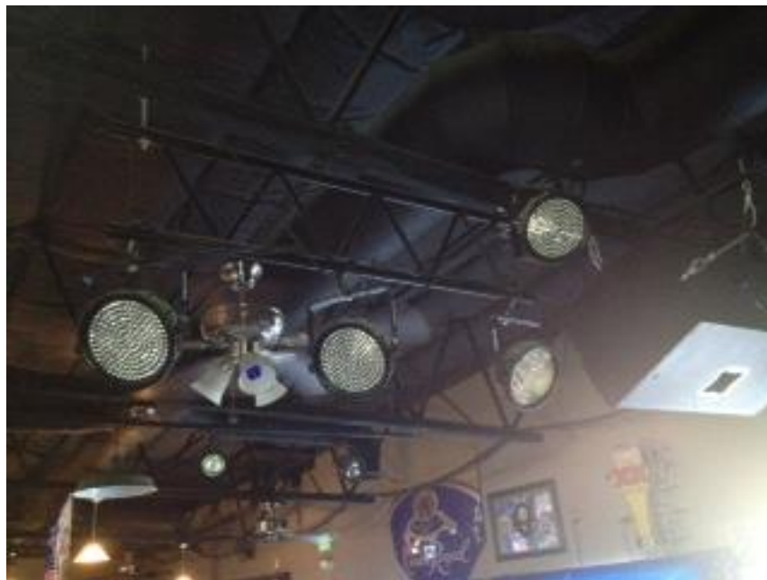
Stage Right Lighting
